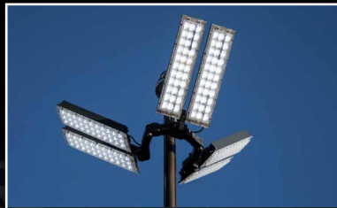
360° area flood lighting
